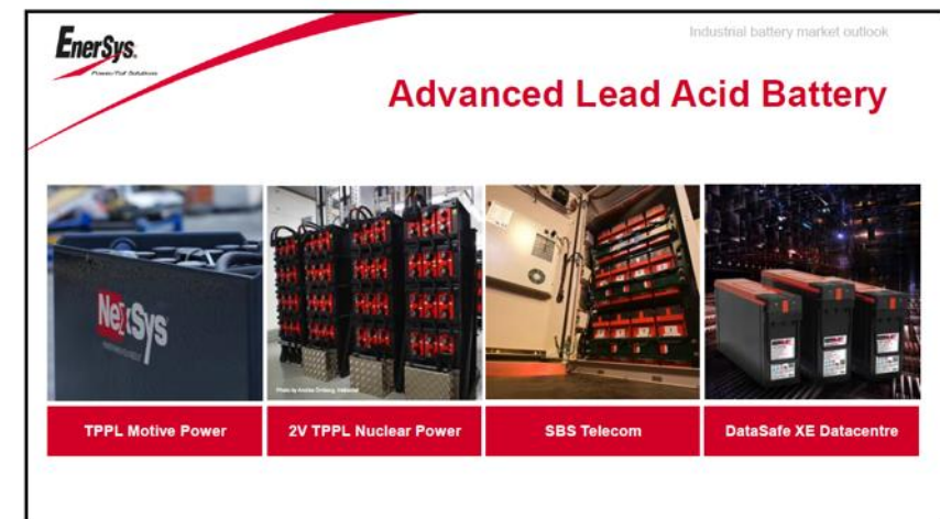
Stationary lead acid batteries in use
