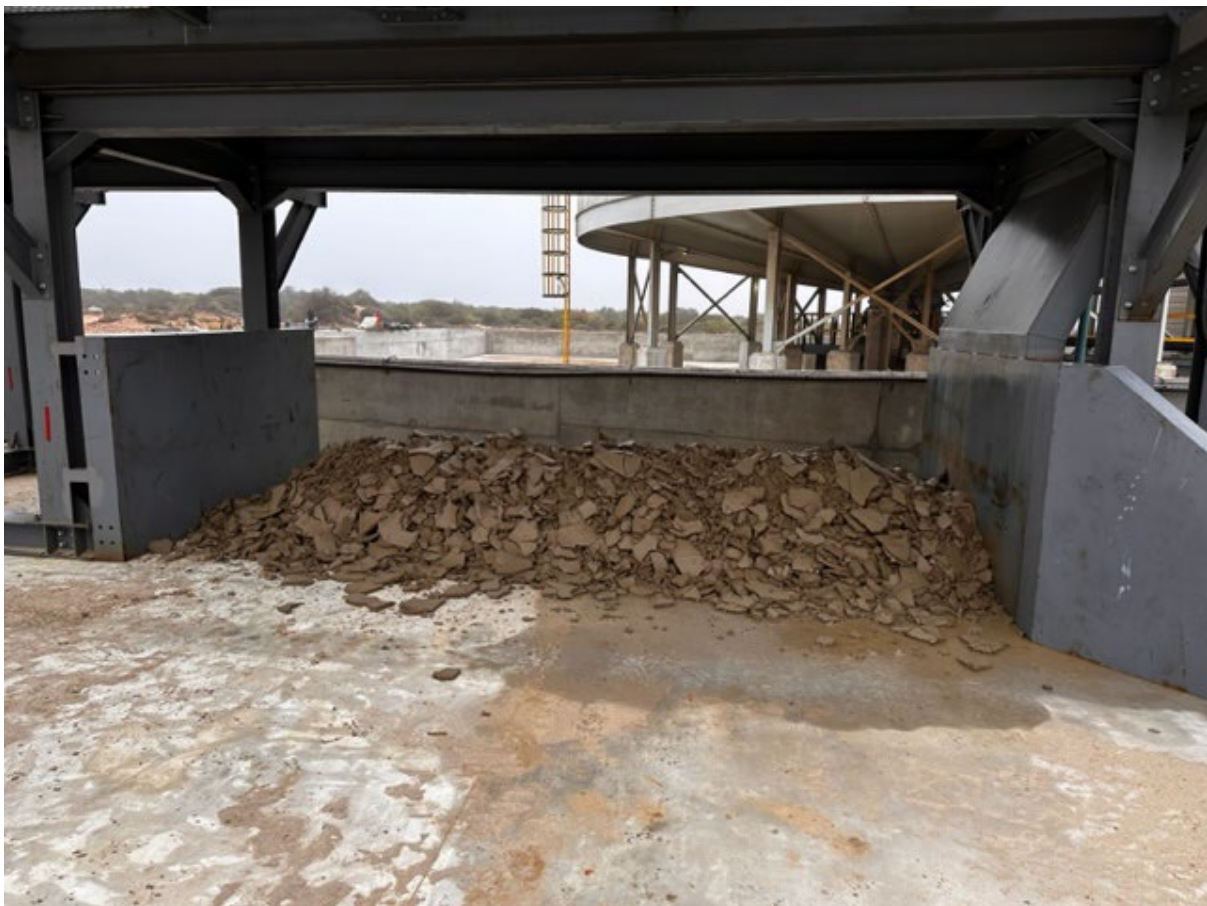
Figure 3 Filtered slimes discharge cake from initial tests. The filter is fed from the thickener (in the background) as an alternative to pumping thickened slimes to the mining void
