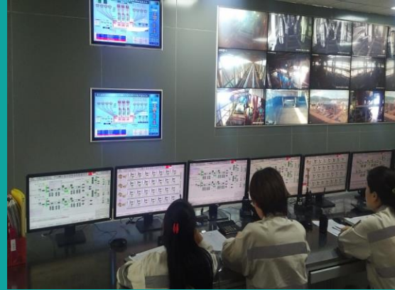
RKEF Control Room
