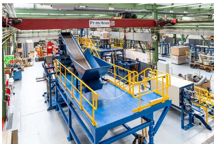
Figure 1 – Two stage Shredding Circuit
