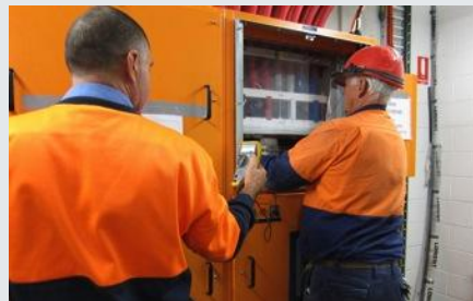
"On Saturday we achieved another significant milestone for our Brisbane B1 Data Centre Site. Power went live."
