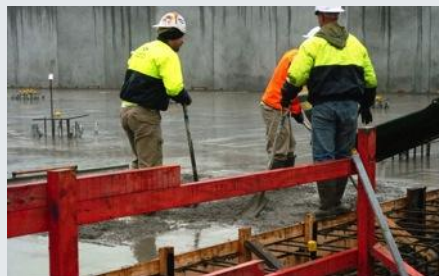
"This morning we finished pouring cement for data hall 3. As you can see it is raining and a balmy 10 degrees!"
