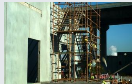
"Each day, more and more of M1 comes together. Above, you can see the scaffolding in place for lift wells 2 and 3."
