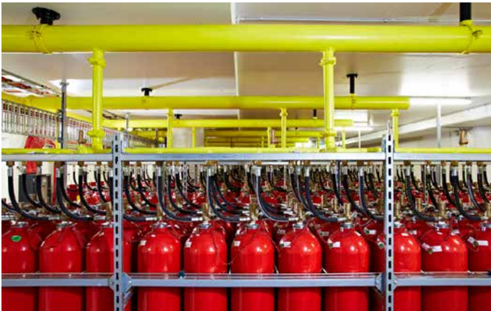
Inert gas fire suppression system
