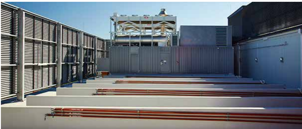
Containerised Piller DRUPS units (P1)
