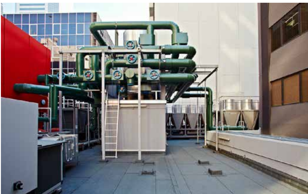
Air-cooled UNIFLAIR chillers (B1)
