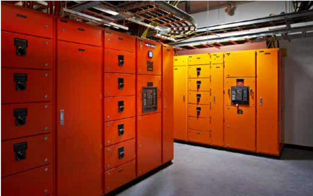
High Voltage switchboard
