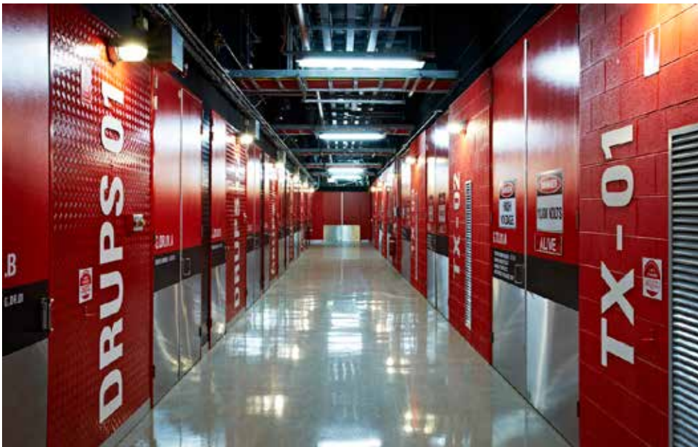
Diesel Rotary UPS corridor (M1)
