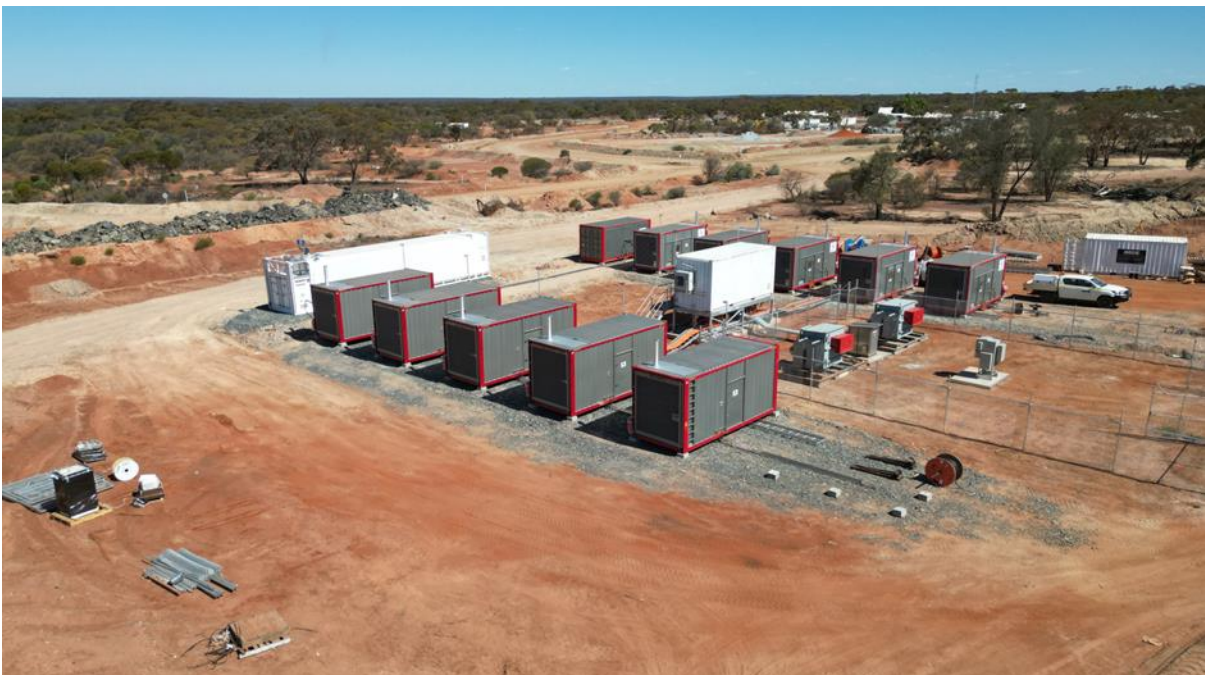
Figure 10 - Aerial view of primary power station.
