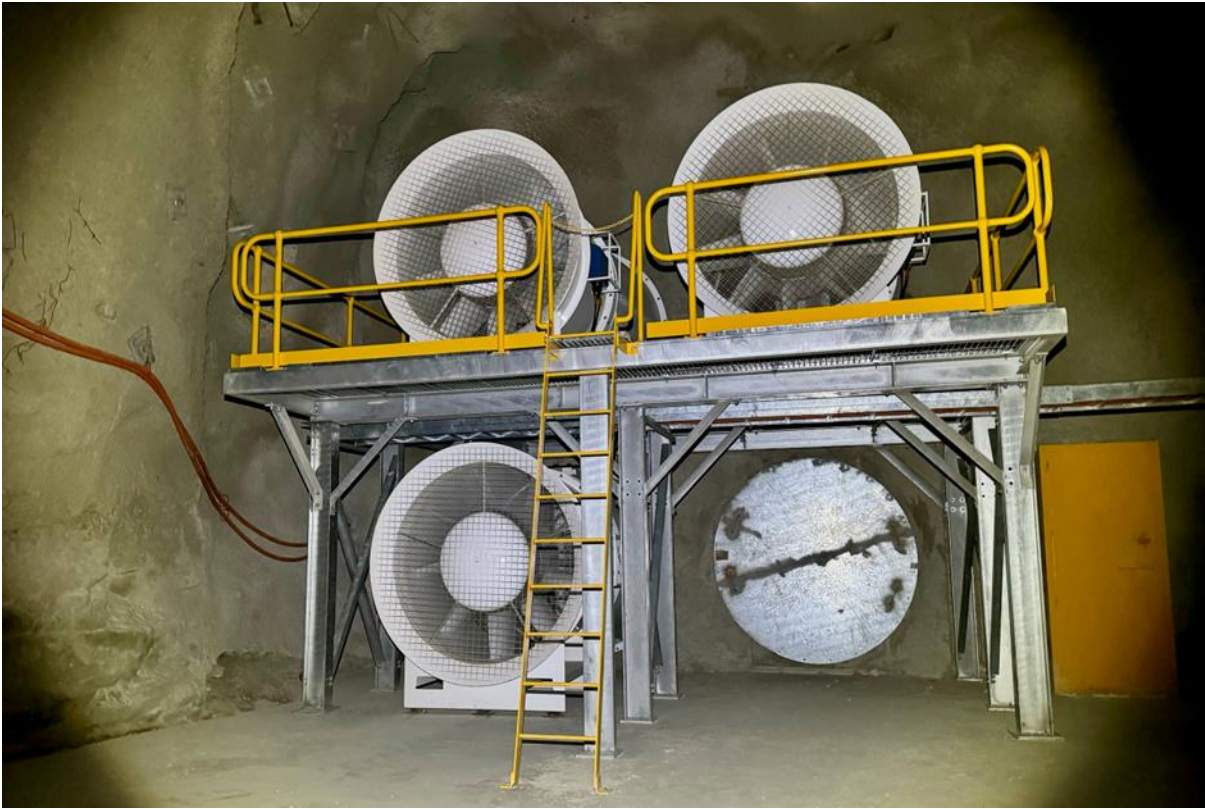
Figure 9 - Primary ventilation fans installed.
