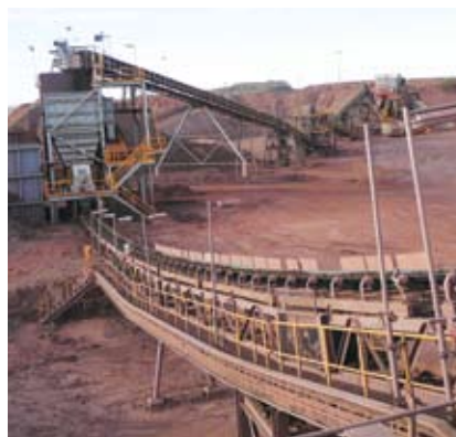
Surge bin and crusher from scrubber feed platform
