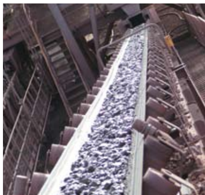
Lump product conveyor to drum circuit
