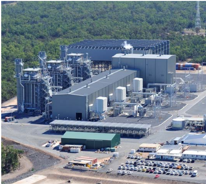
Darling Downs Power Station
