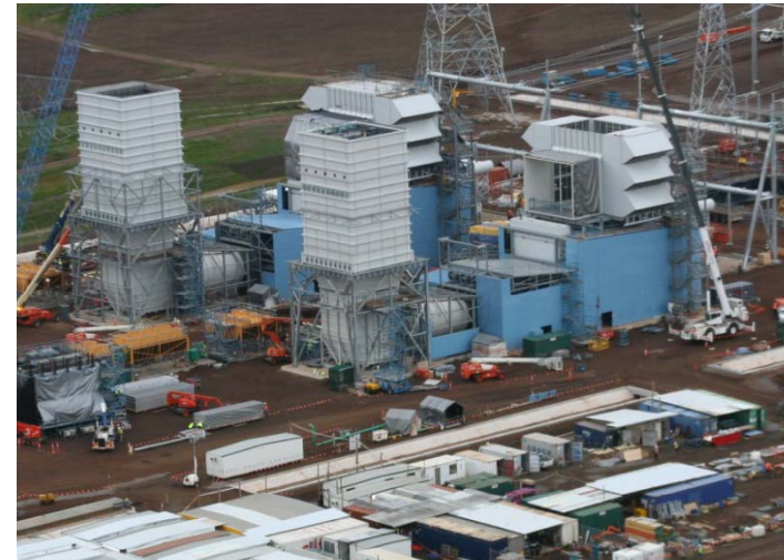
Mortlake Power Station
