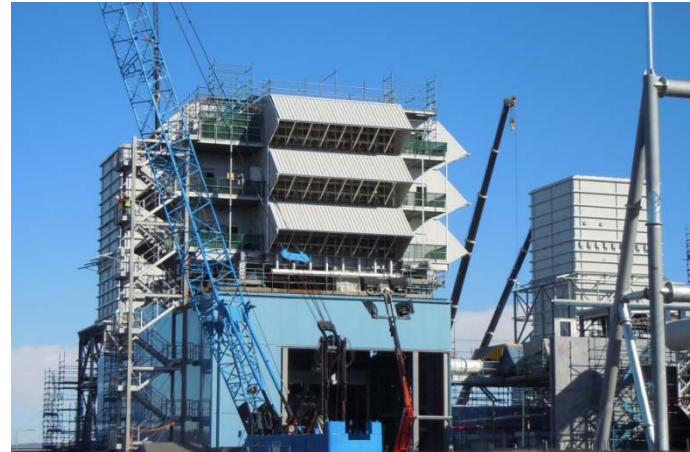
Mortlake Power Station
