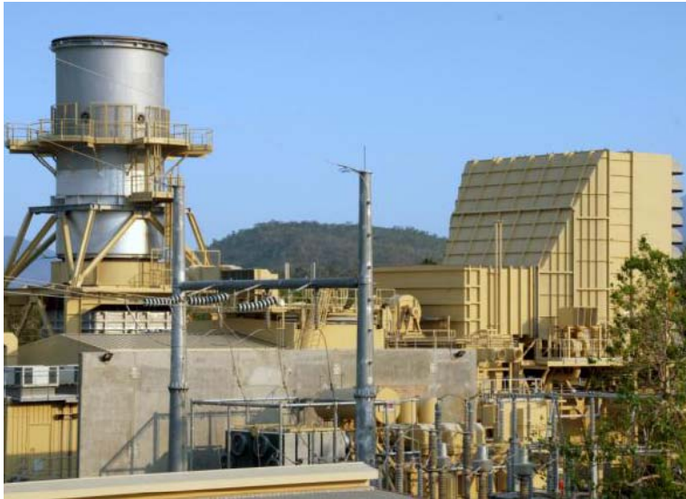
Mt Stuart Power Station
