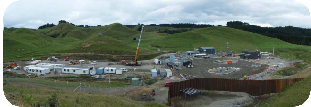
Ahuroa gas storage project
