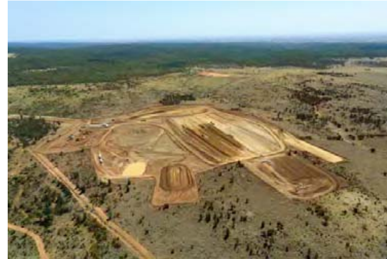
Eurombah Creek – Gas Processing Facility
