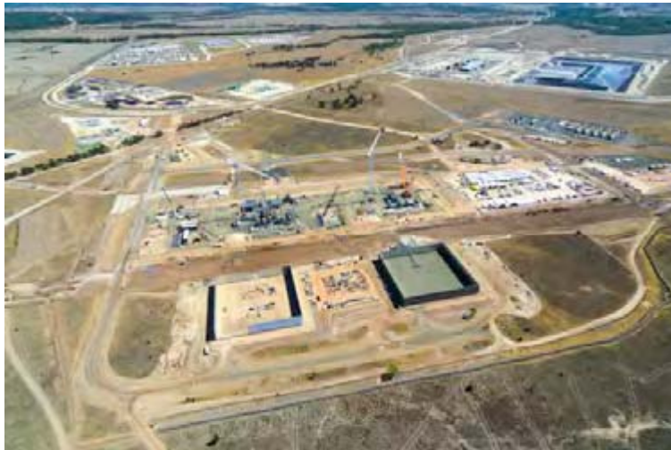
Reedy Creek – Gas and Water Processing Facilities
