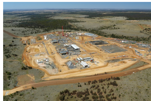
Eurombah Creek Gas Processing Facility
