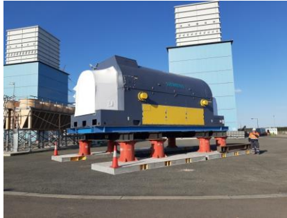
New stator on-site at Mortlake
