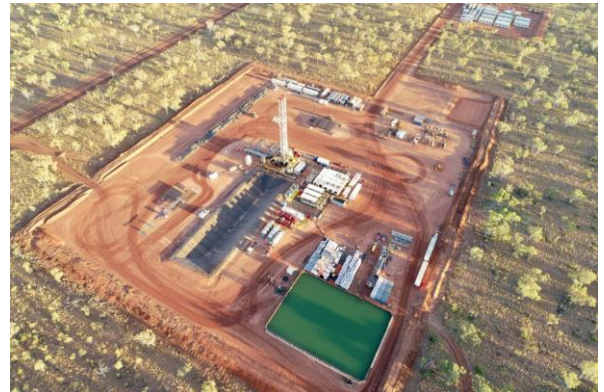
Kyalla 117 well site
