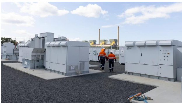
Picture: Eraring battery
