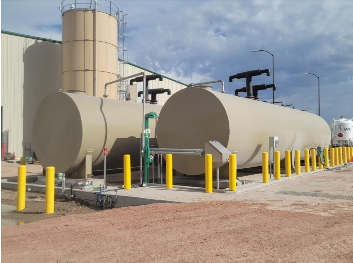
Figure 5: Bulk sulfuric acid storage facilities at Lance
