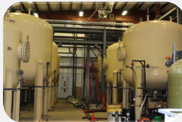
Satellite Plant Ion Exchange System
