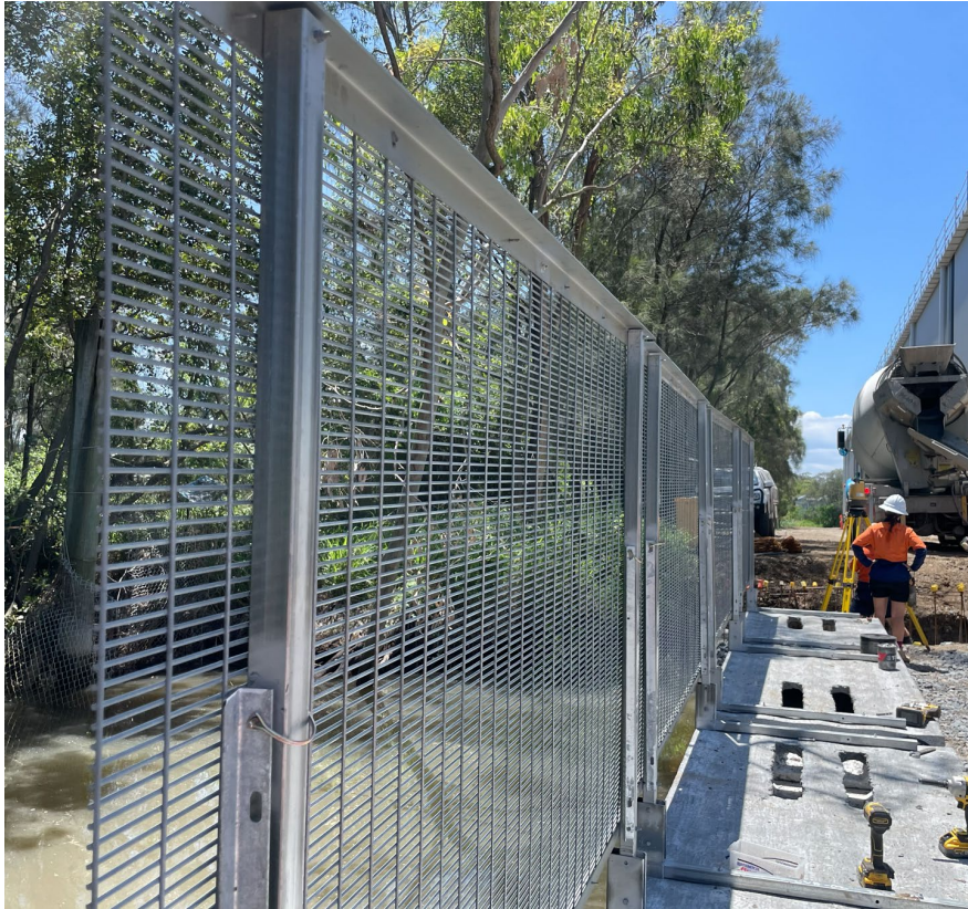
Image 1. Pre-installed PIEPS® edge safety system
