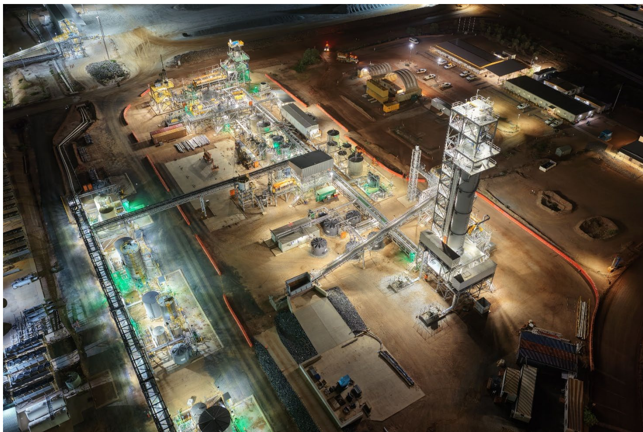
Image: Mid-Stream Demonstration Plant as at 2 April 2026.
