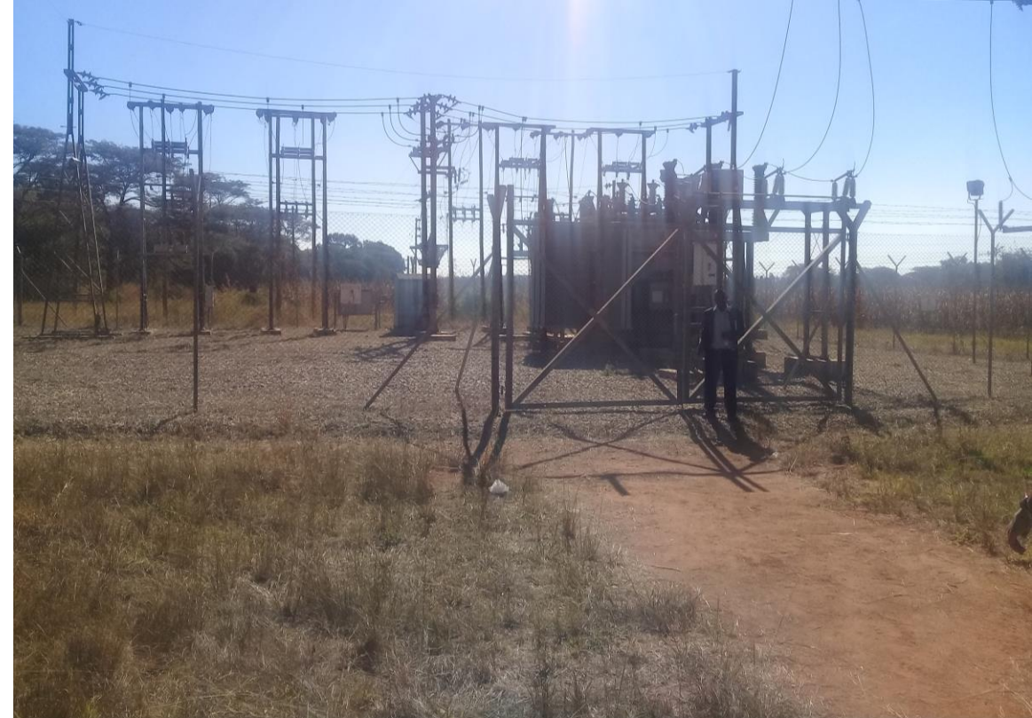
Atlanta substation located approx. 9.5km from Arcadia
