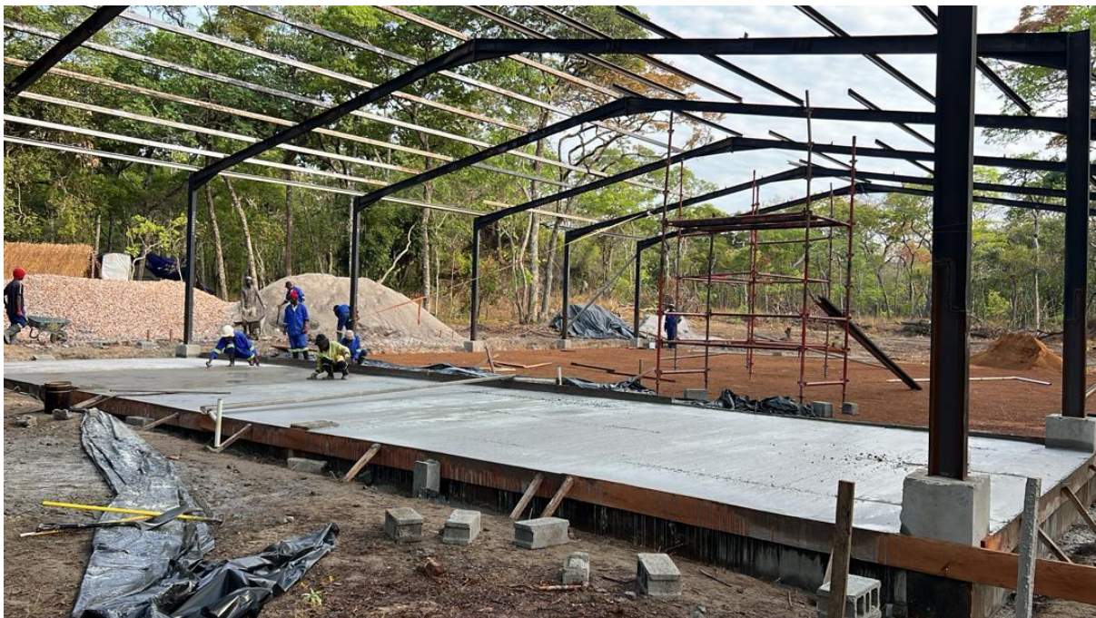
Figure 12: Construction of the Mumbezhi Coreyard is well underway with foundations established and concrete flooring being poured
