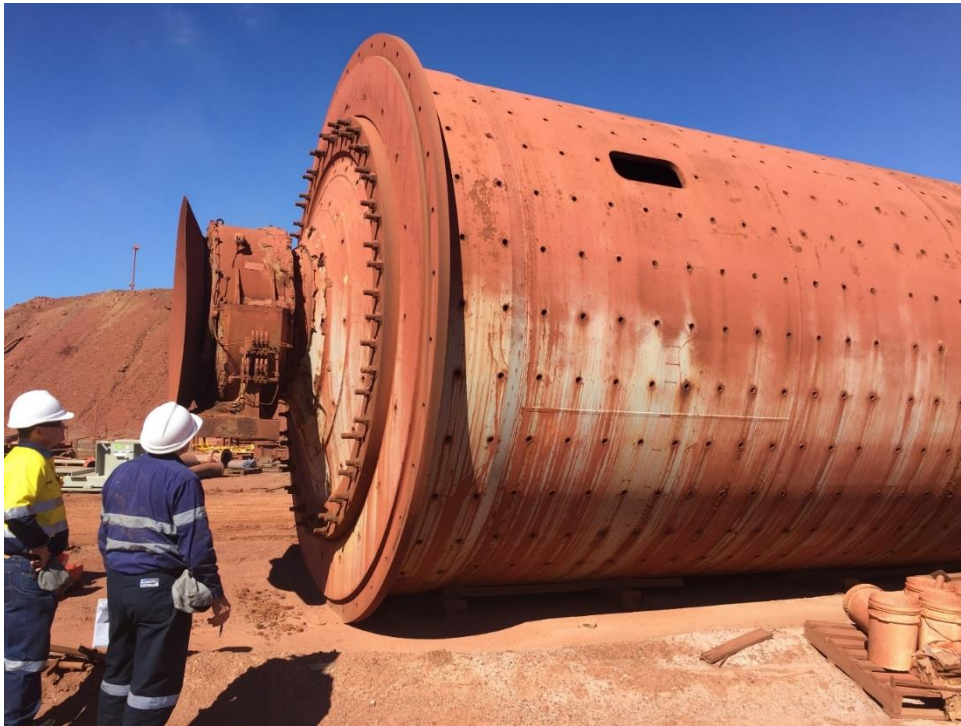
Figure 1. The 2.5MW Ball Mill Shell 60km from LGP
