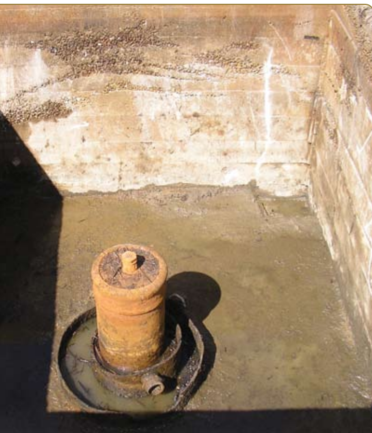
Re-entry well in Geo-Madrid Geothermal District Heating (GDH) Project.
