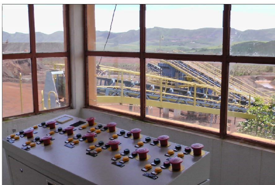
Fig. 4 Processing plant control room
