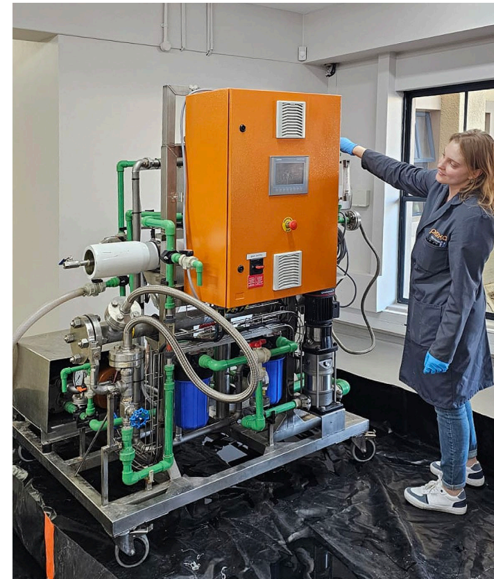
Waste-Water equipment trials, PSG Demonstration Facility
