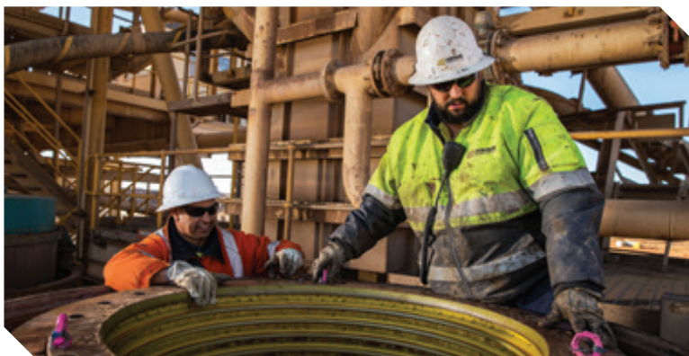
Miller Tamarua and Adrian Groves at the Nelson Concentrator - Garden Well Process Plant
