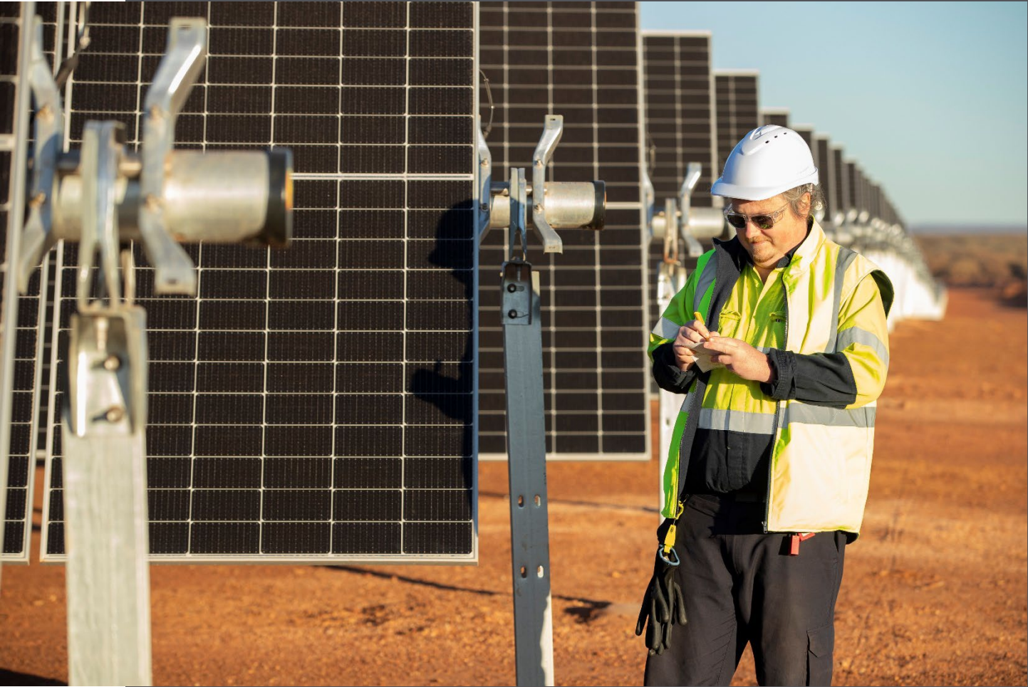
9MW solar farm (Duketon)
