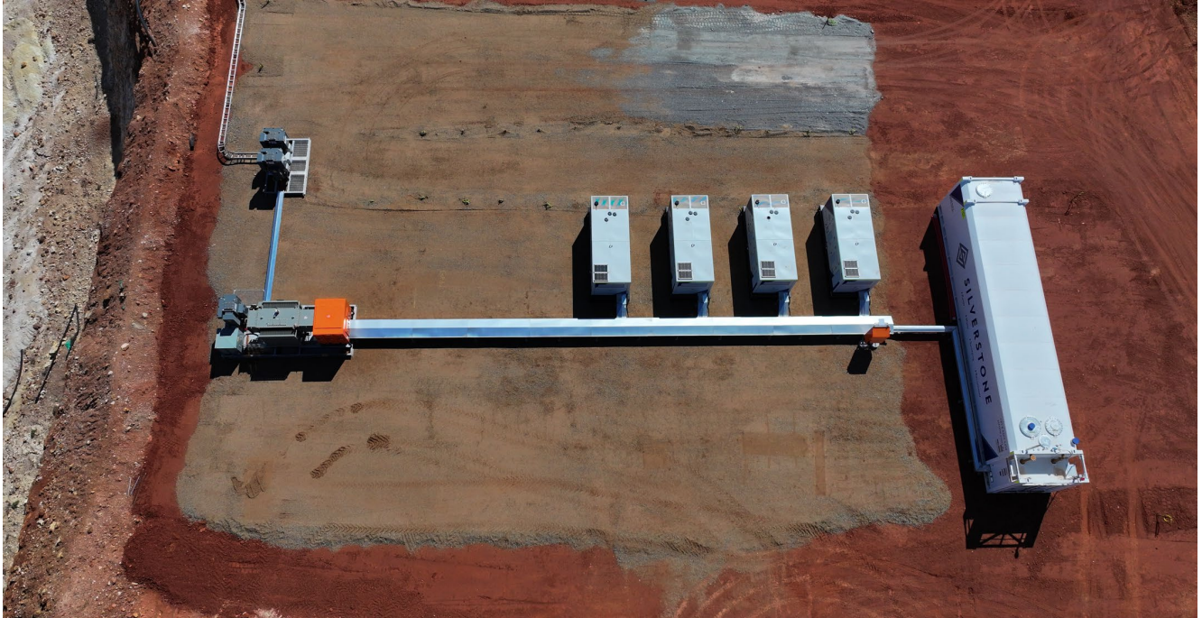
Figure 6 – Main and Pollard temporary power station
