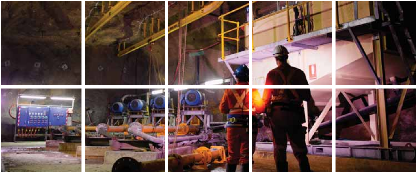
Above: Pumping station, Gwalia underground
