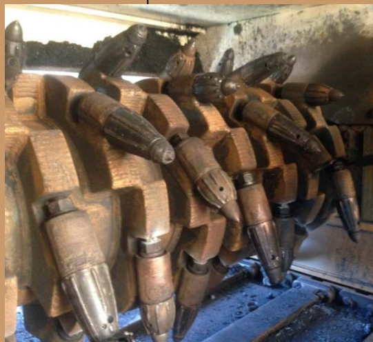
CV01 Fixed Speed Feed Conveyor
