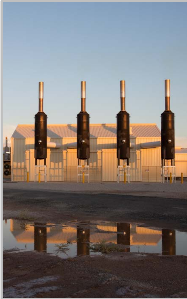
Gwalia chiller plant
