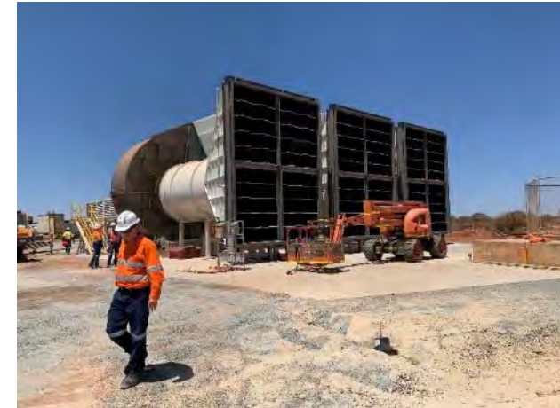
Installation of surface fans at Gwalia
