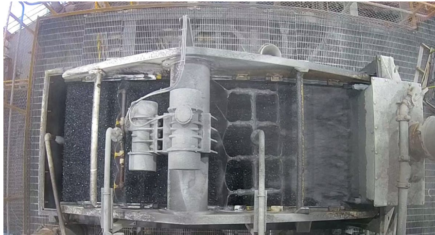
Gravity screen at Touquoy processing plant
