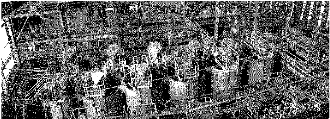
Figure 9: Part of the flotation circuit at the Intec Hellyer Mill, with the SAG and ball mills in the background
