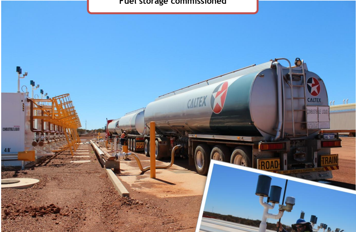
Fuel storage commissioned
