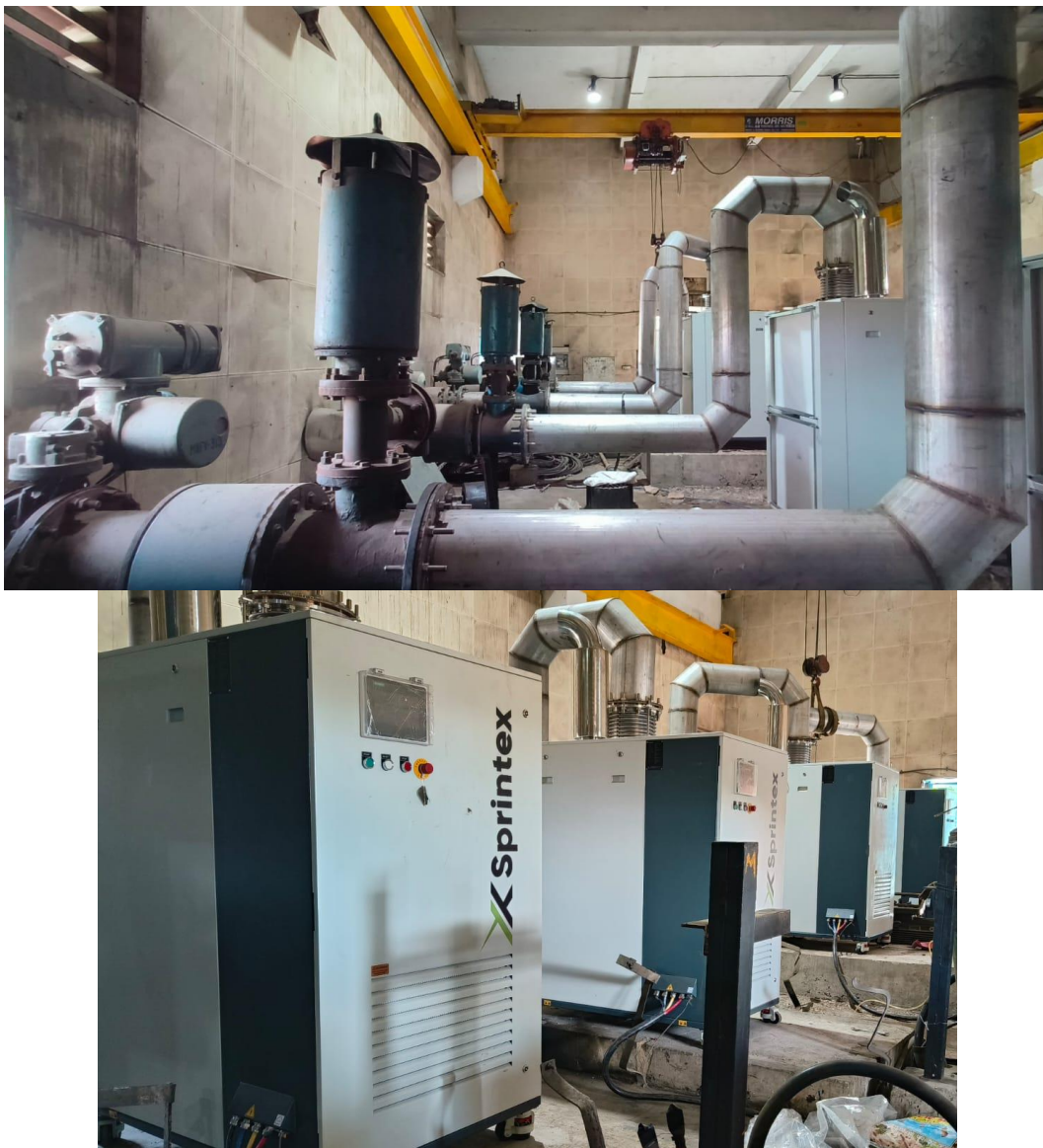
Images: Kondli 45 MGD Sewage Treatment Plant
