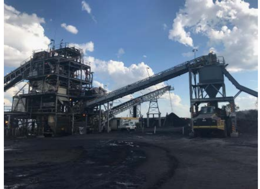
CHPP in operation.
