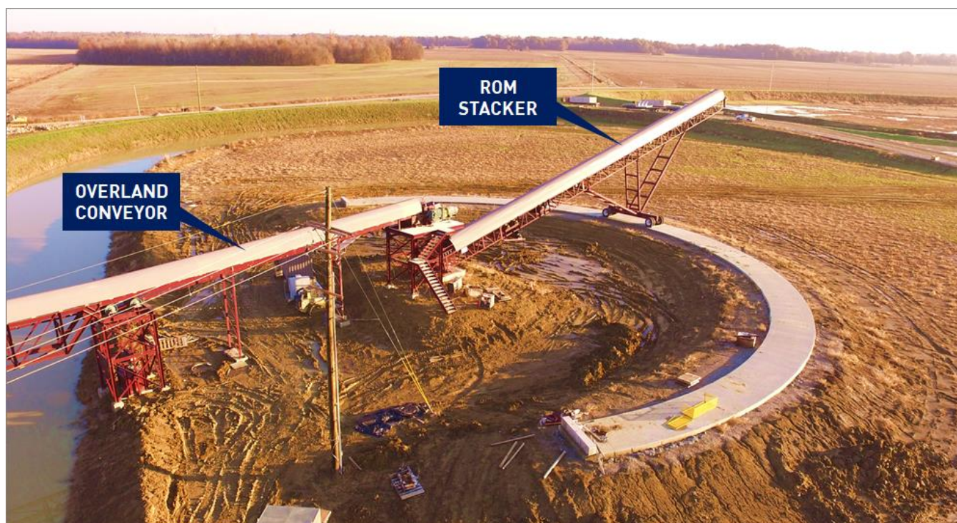
Figure 2: ROM stacker complete and ready to stack raw coal for processing at the CHPP
