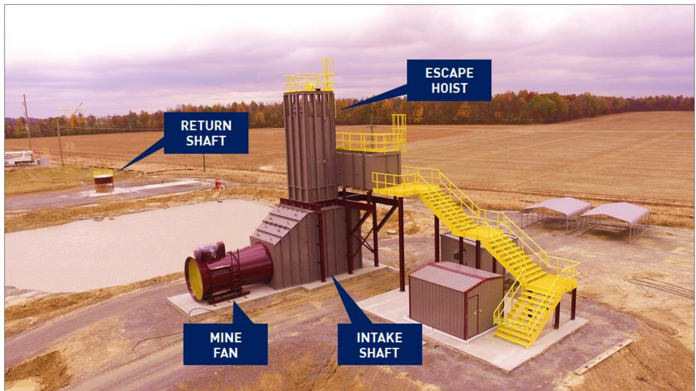
Figure 1: Mine fan, intake shaft and return shaft mechanically complete and ready for commissioning
