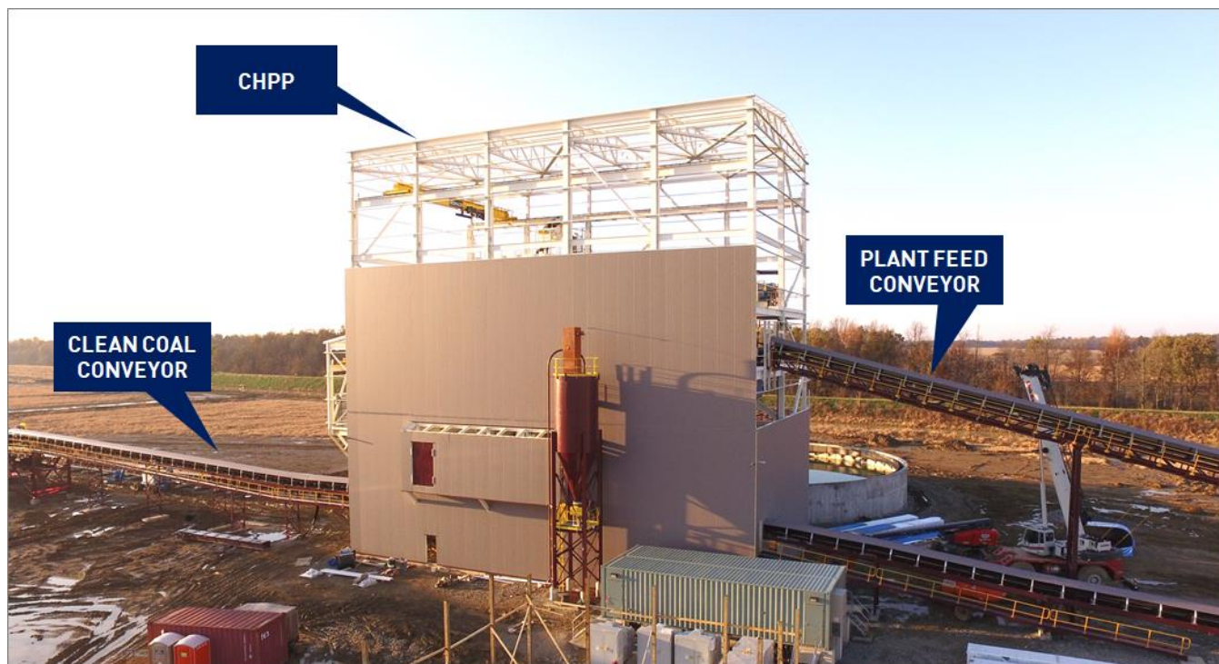
Figure 4: Plant feed conveyor and clean coal conveyor complete at the CHPP
