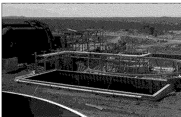
Leach Vats currently installed
