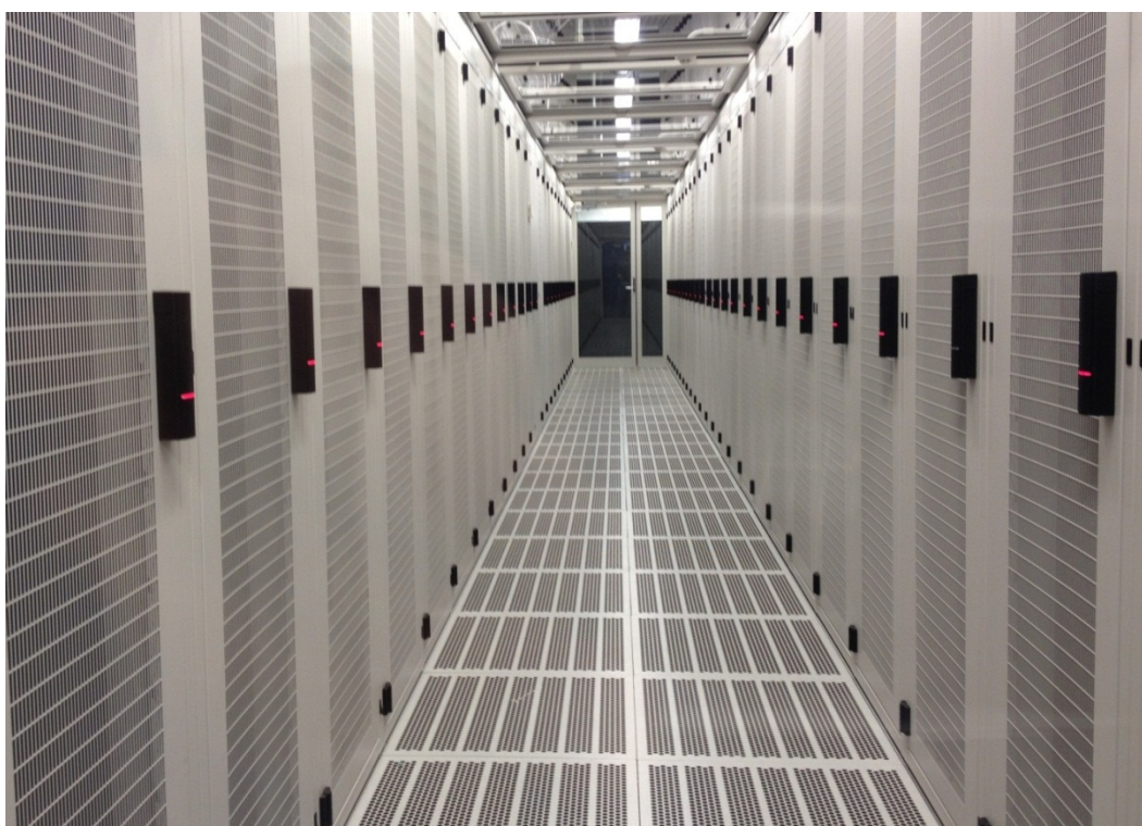
Macquarie Telecom – IntelliCentre 2 Sydney
