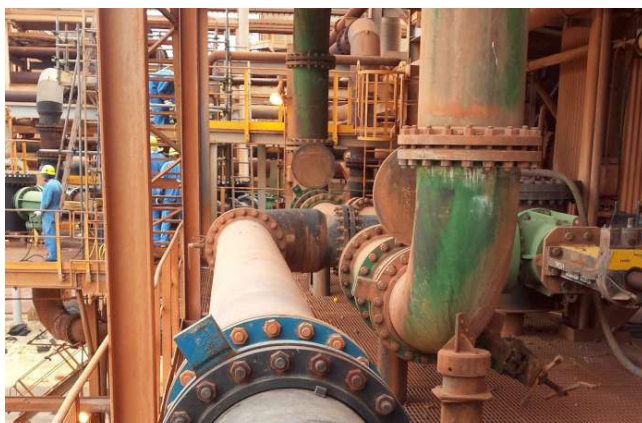
Figure 3: VEEM forever Pipe in-situ (green).
