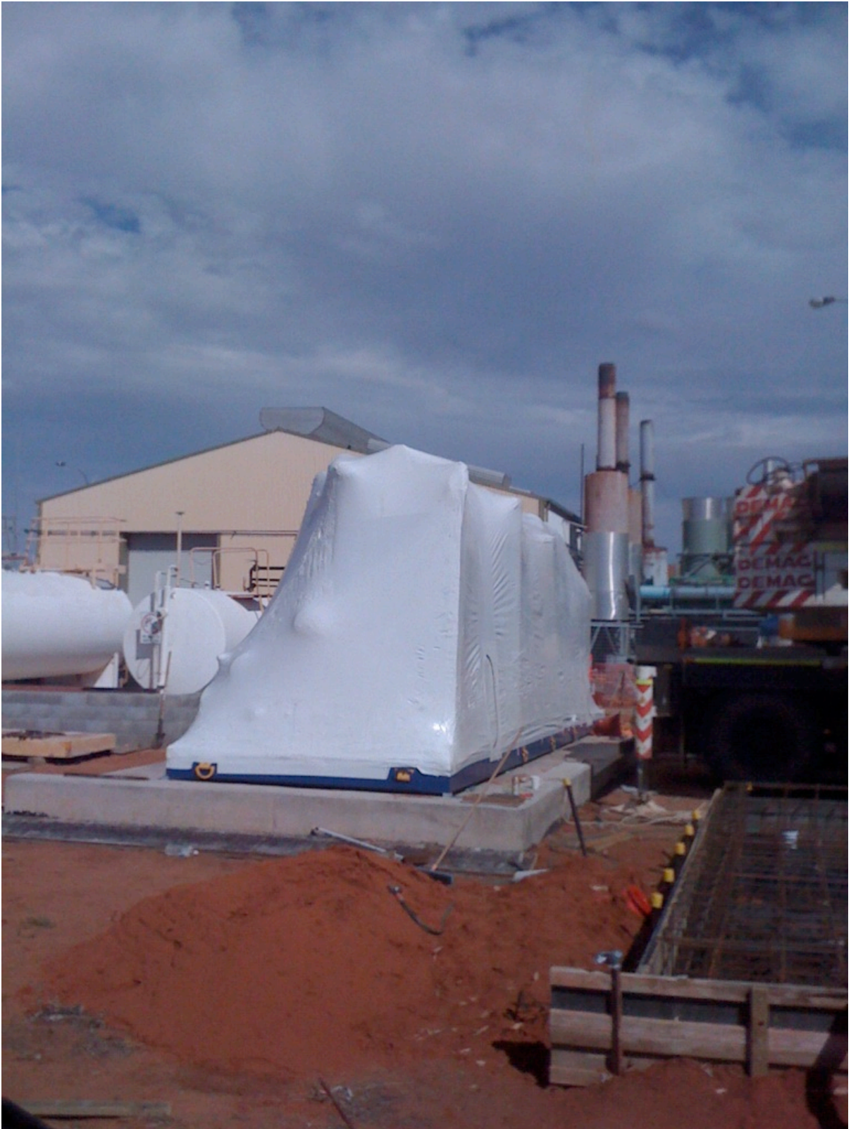
Figure 1 - Enerji's Opcon Powerbox installed on the concrete pad in Carnarvon
