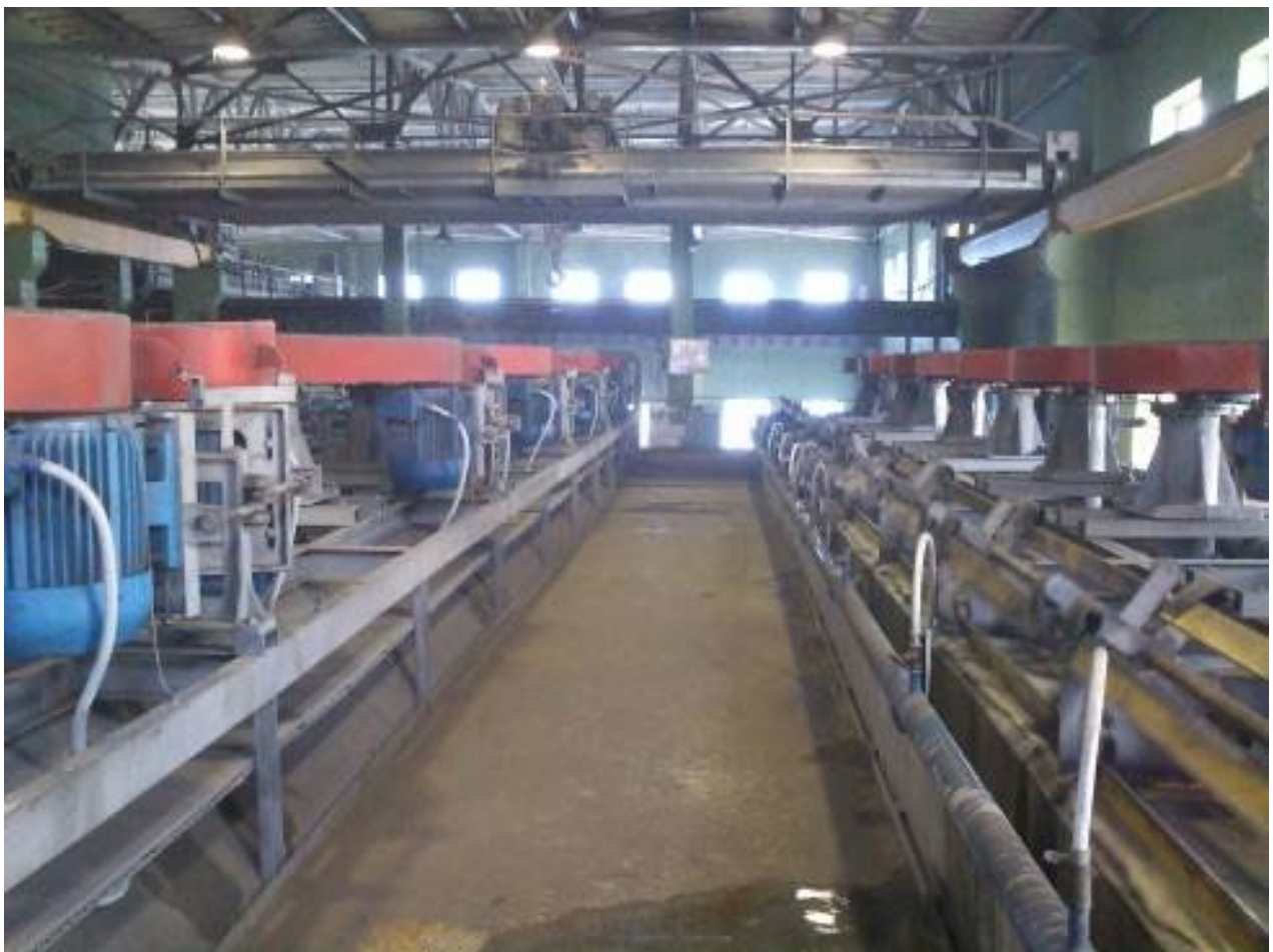
Final stage flotation cells
