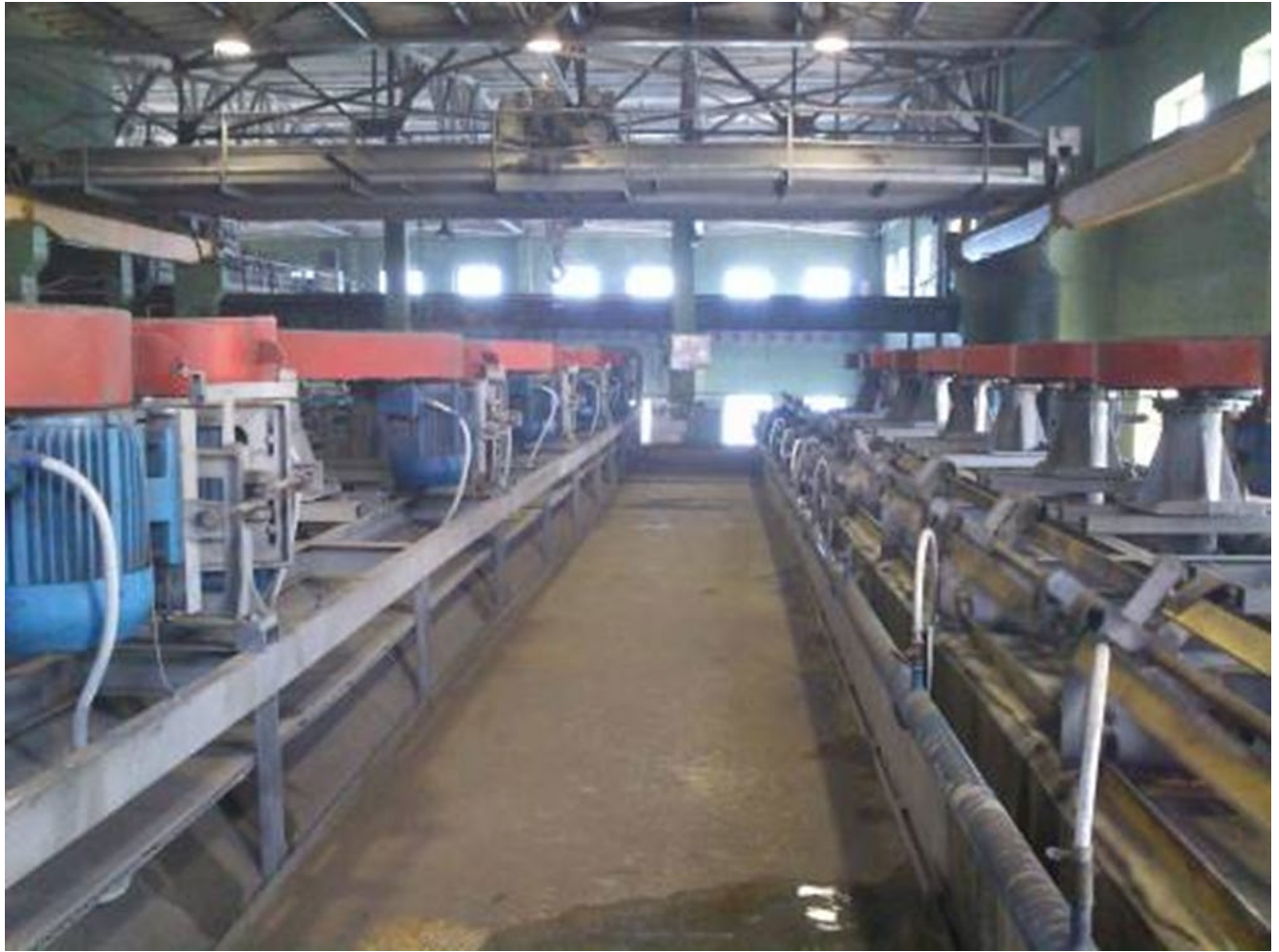
Final stage flotation cells
