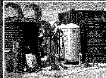
2 x SMDD750 Micron Filters in series installed in a water recycling plant, removing suspended solids and hydrocarbons for a truck washing application. The first filter contains Anthracite and the second filter contains activated carbon.
