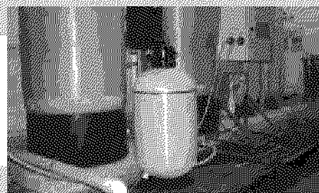
Electronic clarifier brewery installation
