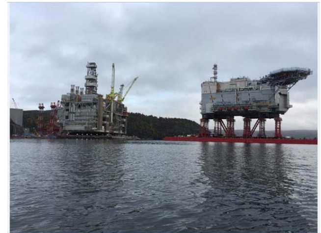
Installation of the accommodation module on the Hebron topsides, Bull Arm, Newfoundland and Labrador (NL)
