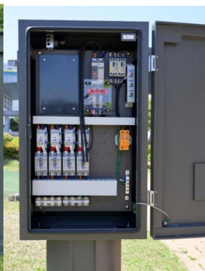
4 channel distribution board
