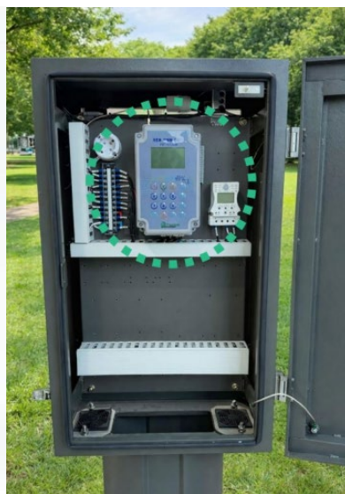
Controller in distribution board
