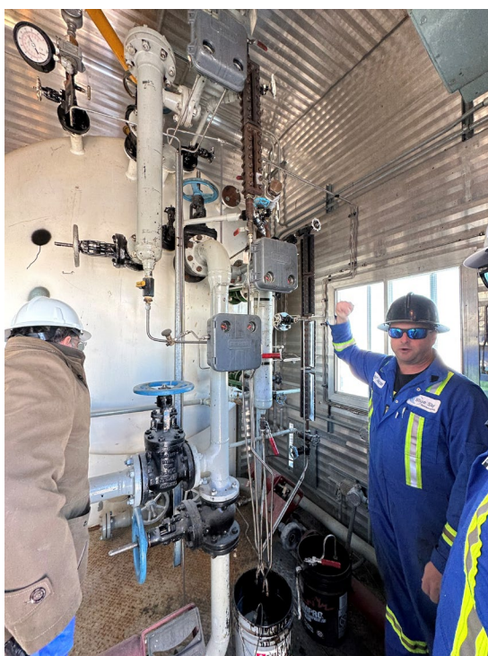
Taber oil treatment facility – Alberta Plains South
