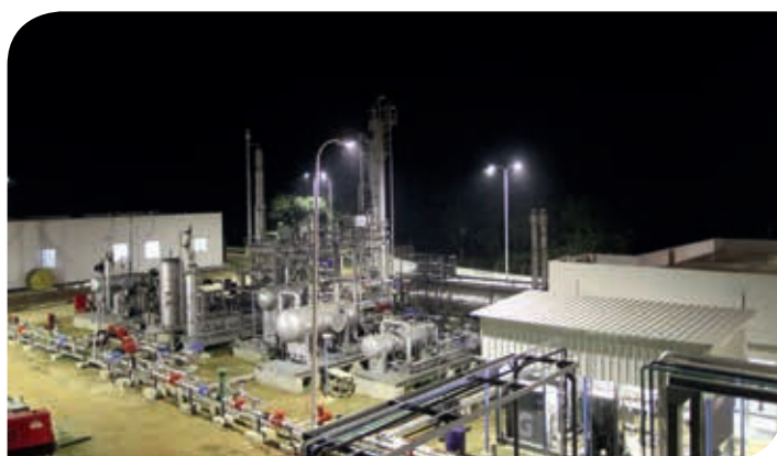
30MMSFD TEG Gas Dehydration Plant
