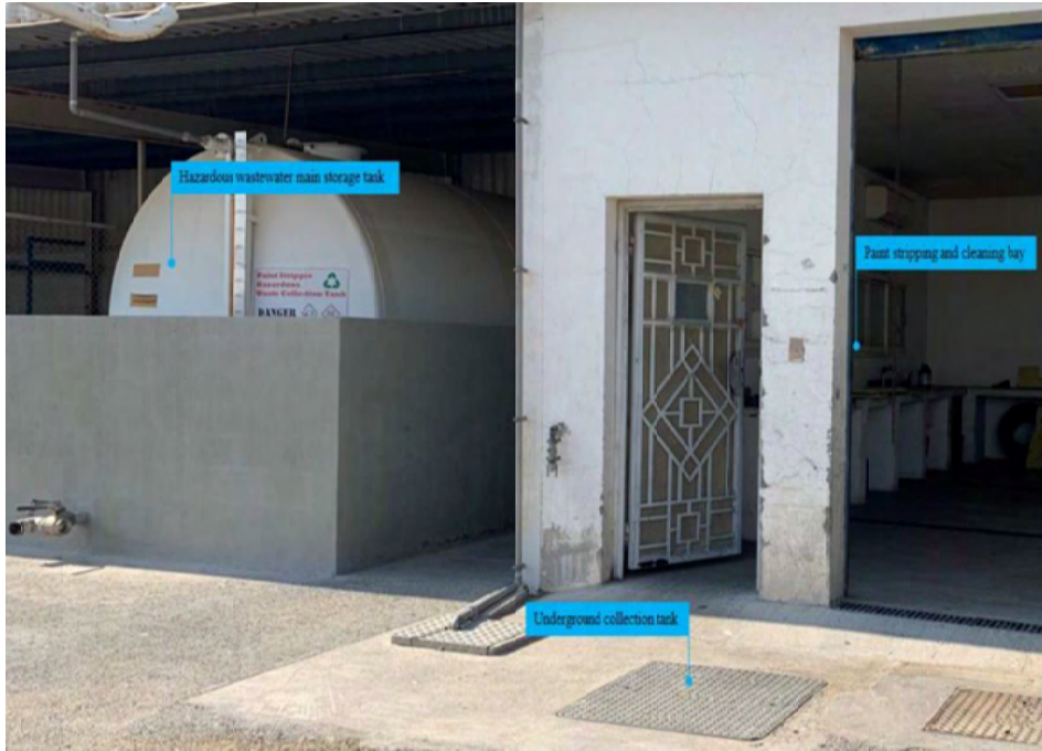
Paint stripping and cleaning facility
